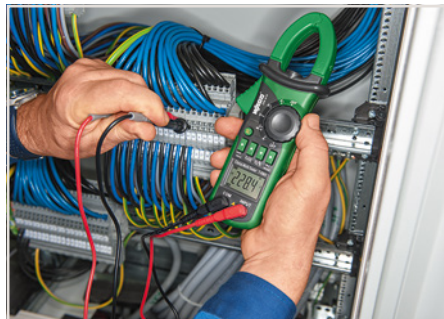
Current measurement in a control cabinet
