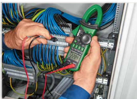
Current measurement in a control cabinet
