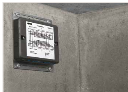
Wall-mounted WINSTA® Distribution Box
