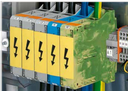
Protective warning marker may indicate: Notice: Power is still on even after switching off the main switch!
