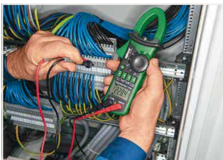
Current measurement in a control cabinet
