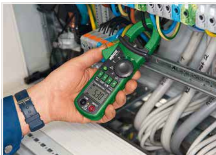
Voltage testing in control cabinet
