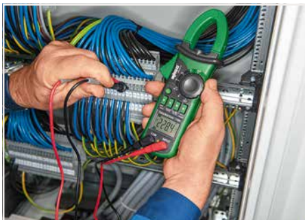
Current measurement in a control cabinet
