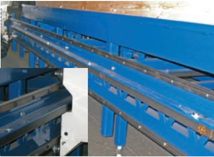
Two nail guns mounted to DualVee wheels and track, travel smoothly and accurately along this 60 ft. wall framing assembly station. The nail guns attach sheets of plywood to 2x4 beams every 16" in one pass.
